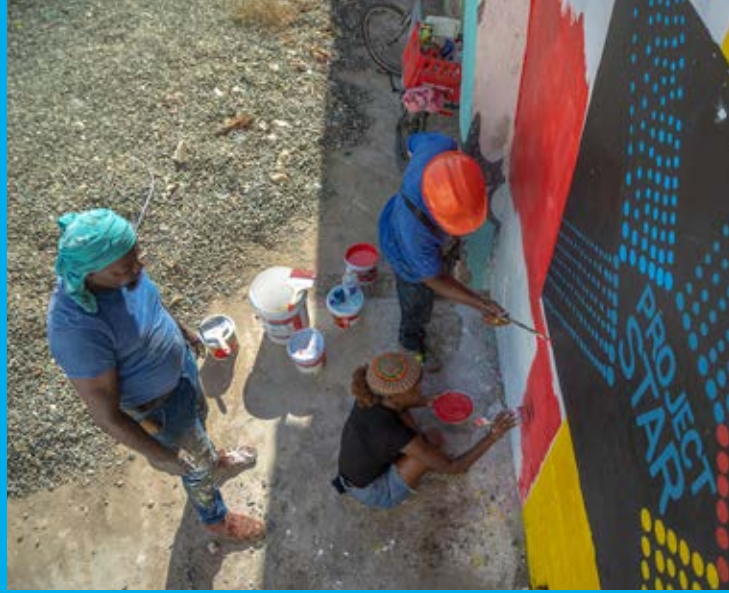
Parade Gardens At the LIFEYARD mural project on Fleet Street in East Downtown Kingston, young people came out to contribute to the larger refurbishment project that is just getting underway. They worked to clear rubble away from the space and started repainting some of the murals.
